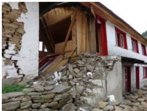
Junbesi School damaged by EQ
