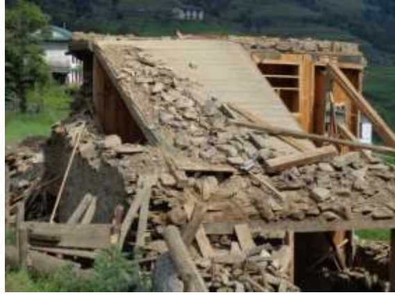
Fully damaged local house of Mapung
