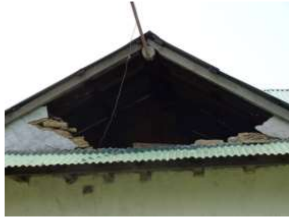
KPHMN – damaged roof
